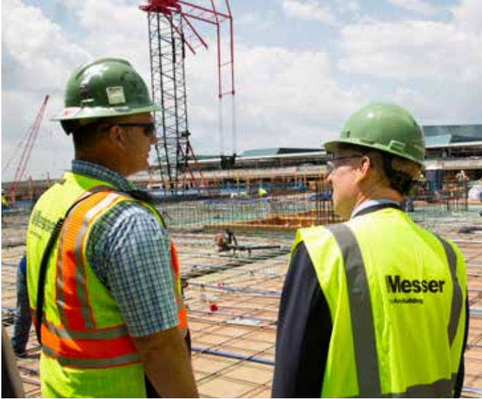
Messer Construction Company carpenter Mark Miracle showcases his company's $114 million design-build project to build a new terminal parking garage and an airport administrative building at the Nashville Airport to Tennessee Congressman John Rose (right).
