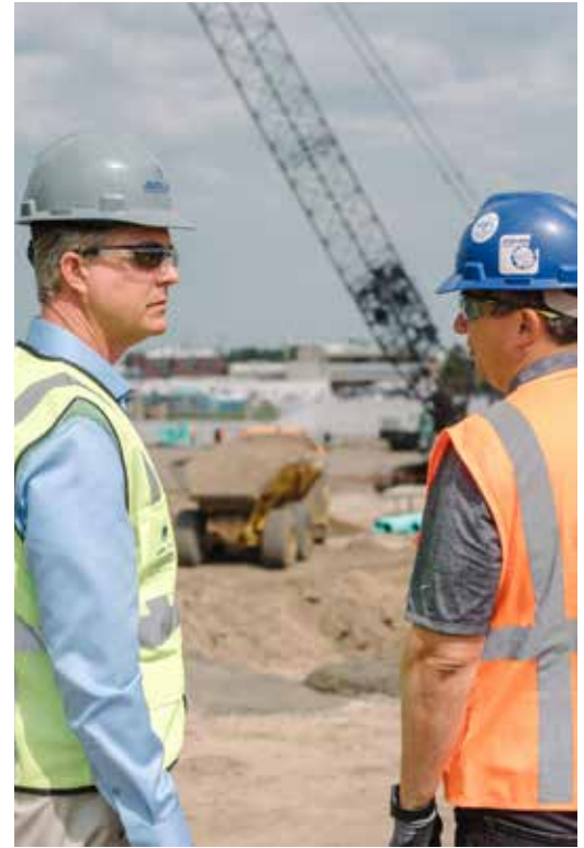
On joint venture project with JE Dunn Construction and Martin K. Eby Construction Co, Kansas Congressman Roger Marshall (left) gets a first-hand look at the construction of a minor league baseball stadium in Wichita, KS along with JE Dunn Vice President Scott Sherry.
