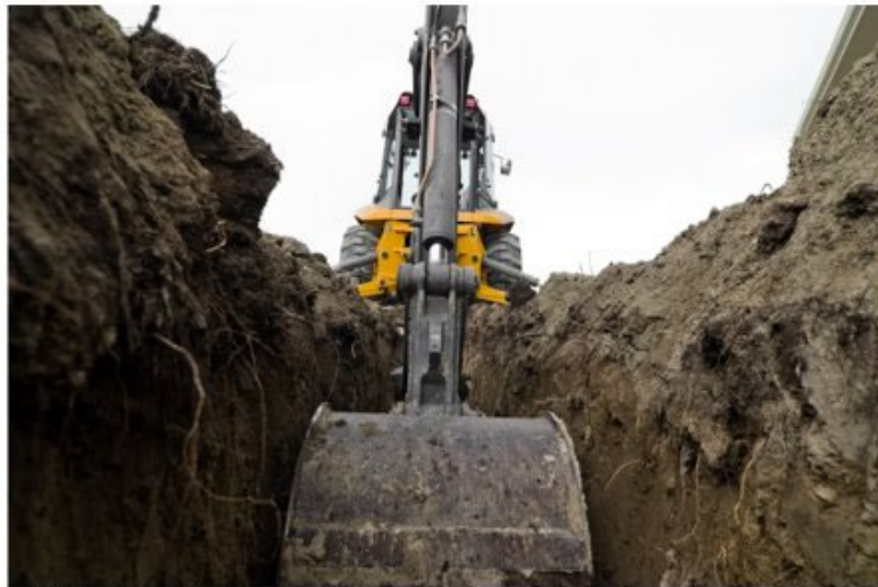
The fatal collapse occurred less than three weeks after the company had been cited for trenching violations on another
