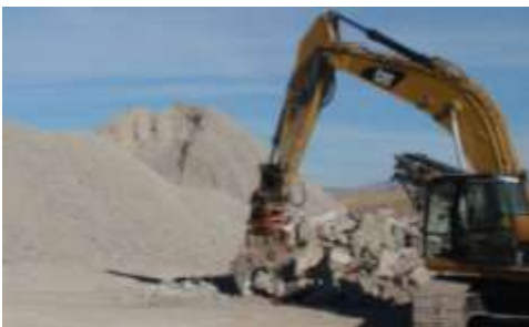
Ames Construction Photo: Metal is being separated from concrete and also being broken up into smaller workable chunks. Note the stockpile of processed concrete in the background ready for direct use or mixing with rock/sand aggregates.
