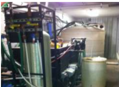
Lane Construction Corporation Photo: Prior to re-use, equipment wash water is treated using clarifying agents for sediment, an oil water separator for oils, and a large carbon filter for other residual pollutants.
