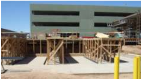
Kitchell Contractors Photo: Use of loading deck for recycling at Kitchell project.
