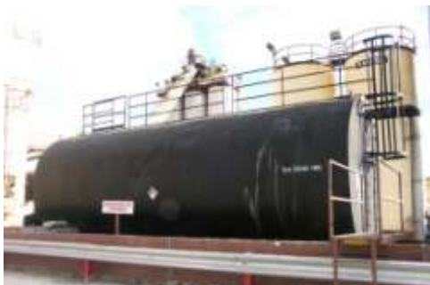
Ranger Construction Industries Photo: Close-up of the burner fuel tank. Ranger sends out used oil for re-processing and then purchases filtered and tested used oil ensuring it meets the regulatory requirements. Ranger uses that product as a fuel for drying aggregate prior to mixing with liquid asphalt to produce paving mixtures. This facility burns about 300,000-500,000 gallons of recycled oil each year.
